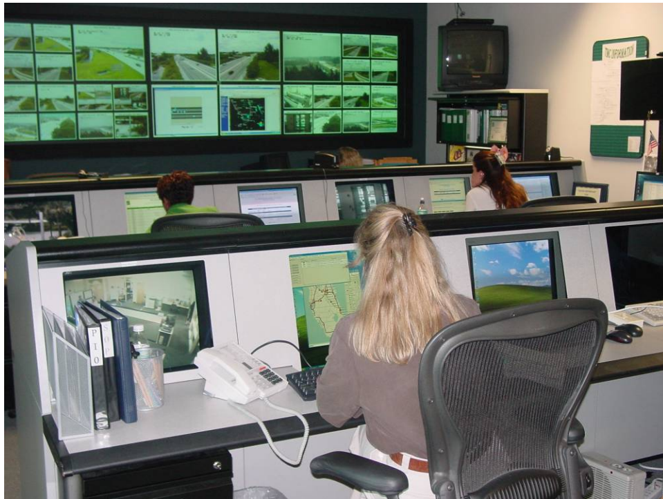
Figure 2 Florida's Turnpike Enterprise Pompano Beach TMC Facility
