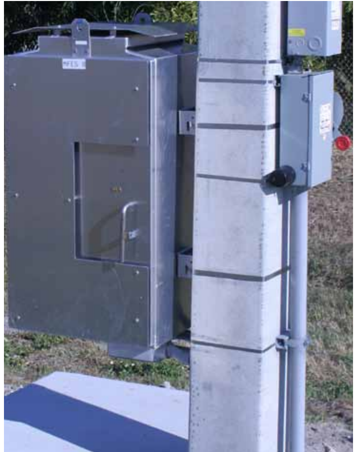
ITS field cabinet, transformer & disconnect
